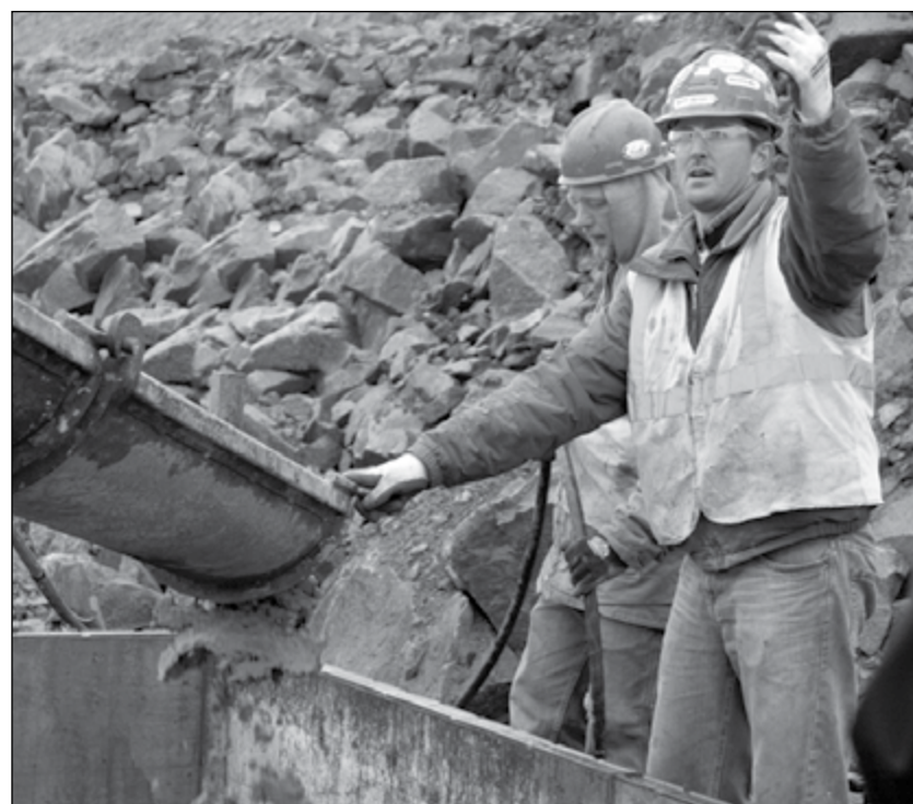
Pouring the first footings at the site of the Essar Steel Minnesota Plant.
