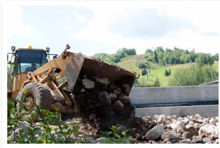
Rip-rap is put in place around the abutment for the Mesabi Trail bicycle and pedestrian bridge.
