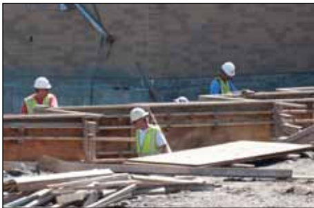
Workers prepare forms as part of the expansion at the Mesabi Community & Technical College in Eveleth.
